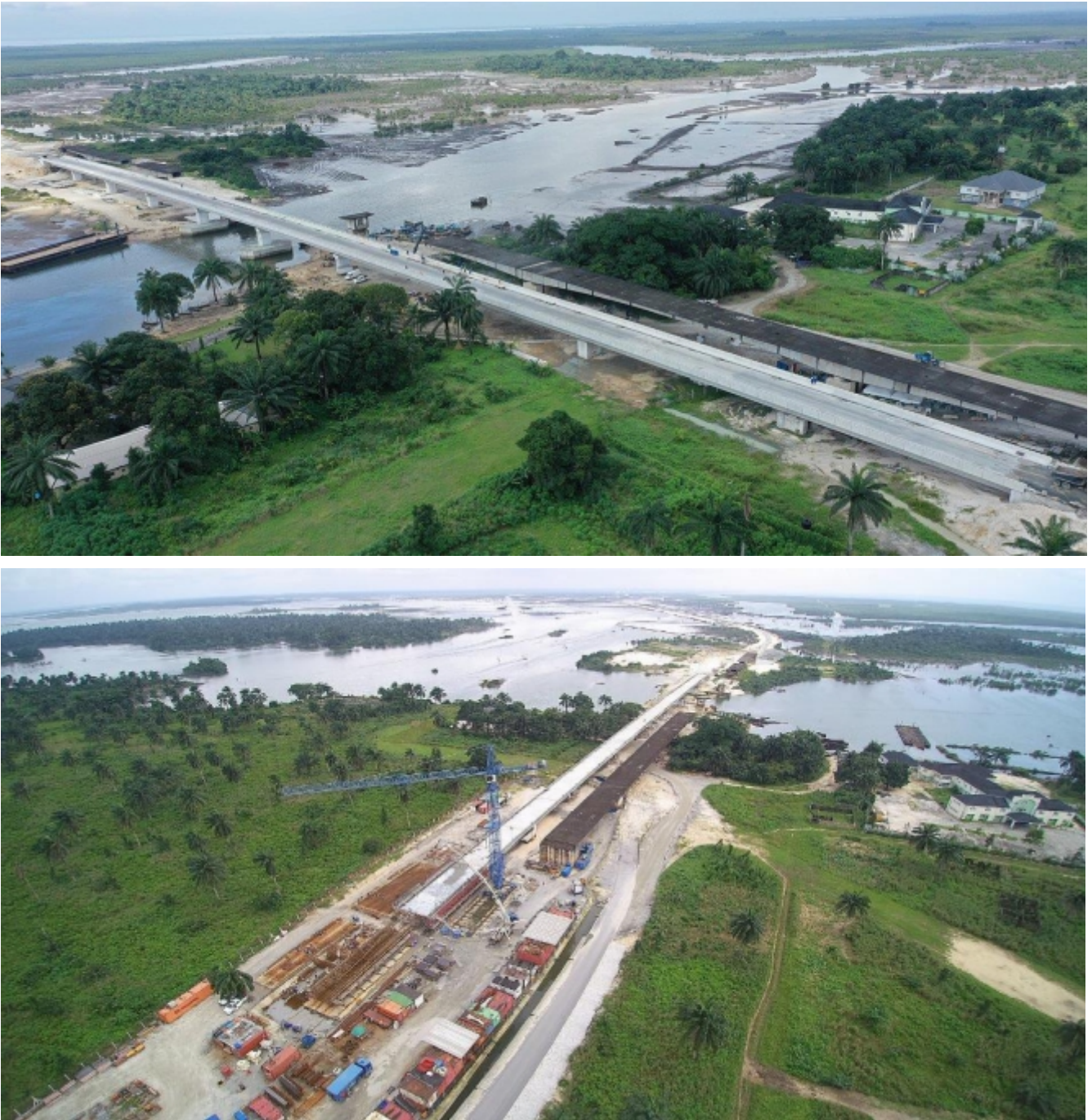
Figure 19: Bodo-Bonny Road under construction and due to link the LGAs of Tai and Khana
